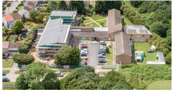
An aerial image of the 30-bed development (left) at Diamond House, Leicestershire.
