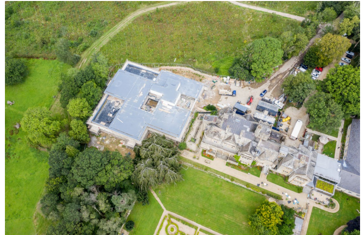
An aerial photograph of the new care home development at Freeland, Oxfordshire.
