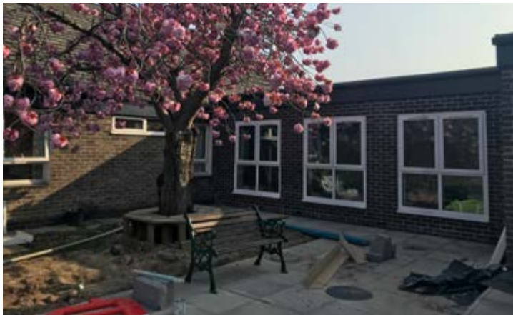
New single storey lounge with improved resident access to landscaped courtyard at Garswood, Wigan.
